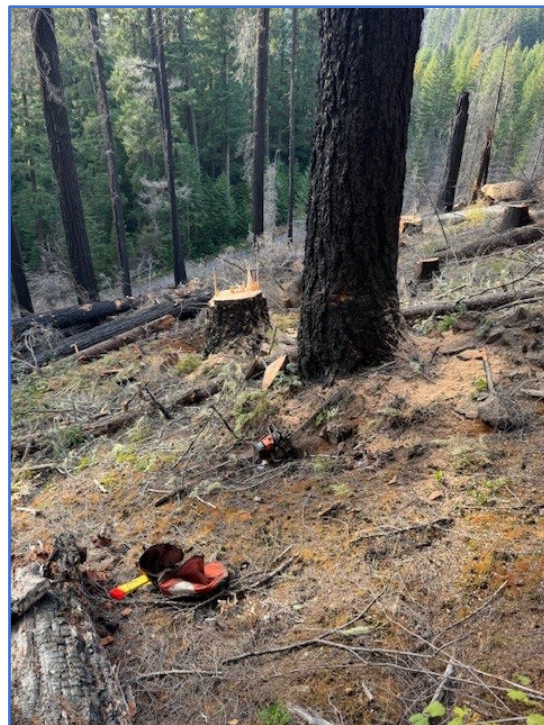
The standing 36-inch diameter Douglas fir tree in the foreground is the tree in which the kickback occurred and injured the sawyer. Note the U.S. Forest Service road at the base of the hill.
