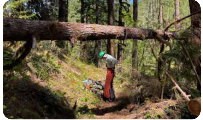
Paul getting ready to work on clearing the stock Ford at Rule Creek (upper skok).
