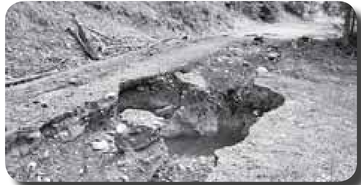
Access to Lambert Creek Horse Camp was made difficult after Forest Service Road (2056) was washed due to the rain and snow melt.
